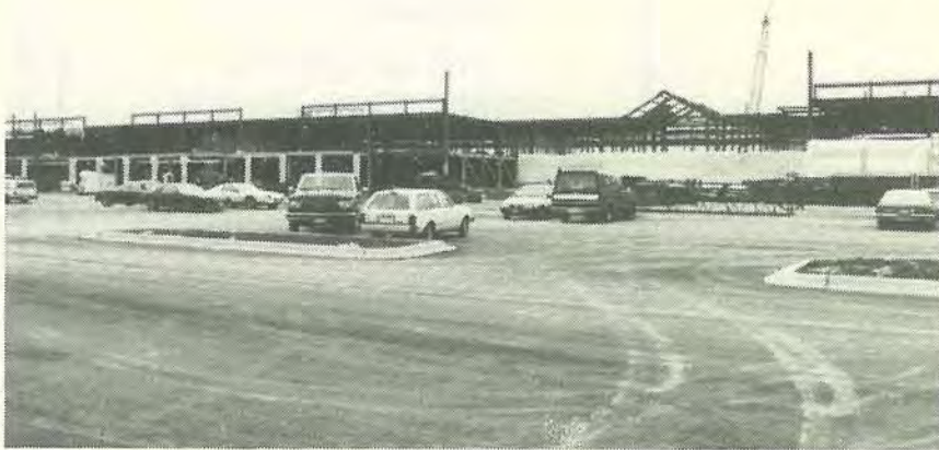
One Schaumburg Place, shown here under construction in February of 1991, is the second largest retail structure in the Village with over 750,000 square feet of floor area. Ultimately, the development is planned to include a twenty-two story office tower and a 400-room hotel.
