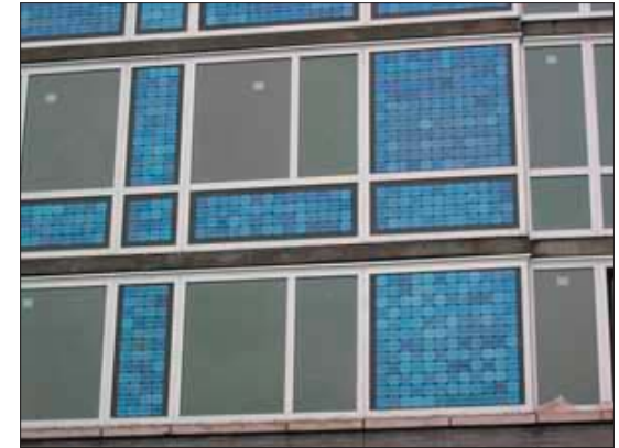
Photovoltaic array on walls.
