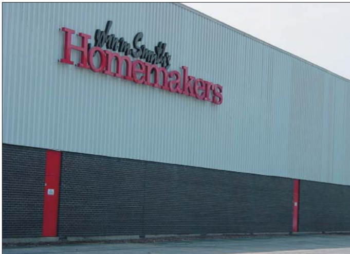
Wall lacking sufficient articulation.
