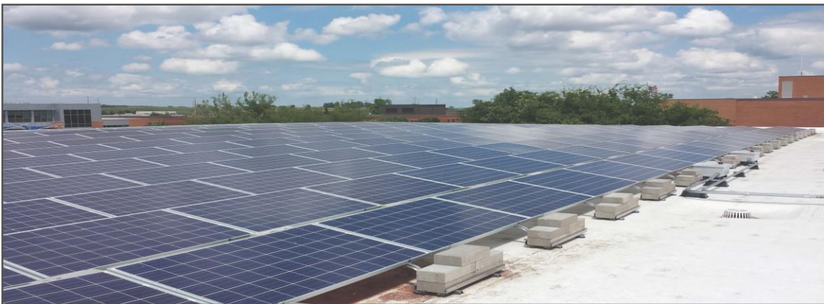
Southwestern Illinois College, 125kW, IGEN
