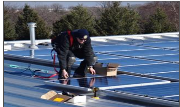
Rooftop Solar, Parkland Community College, IGEN
