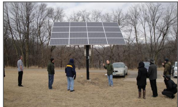
Ground Mount System
